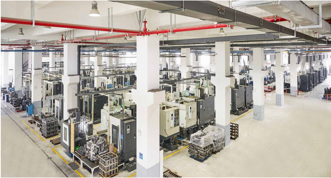
10条机壳机加工半自动线、 10 semi-automatic casing machining lines,
